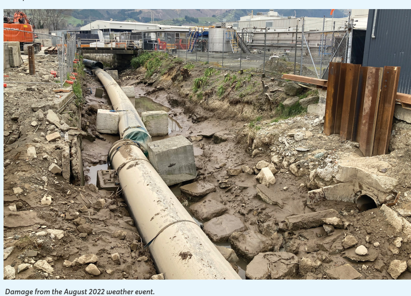
Damage from the August 2022 weather event.
